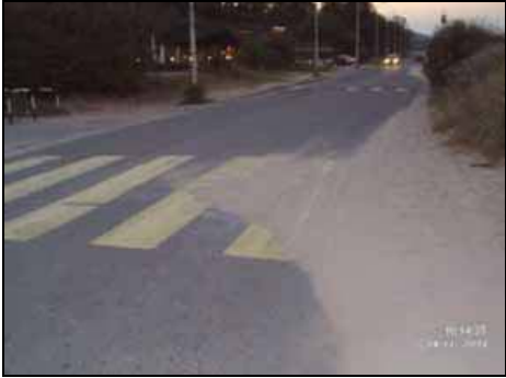
Loose dirt on the carriageway.
